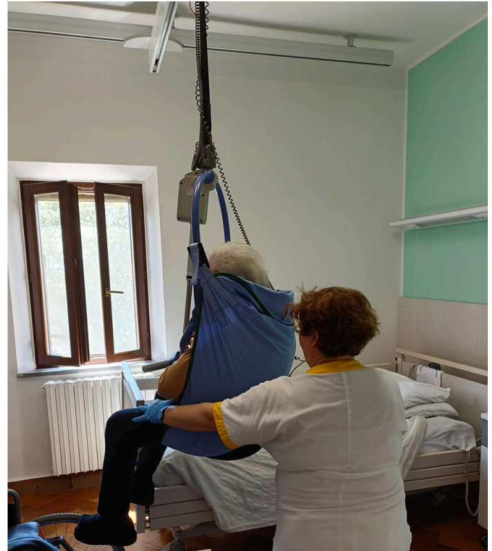
We have 12 beds with ceiling lift to facilitate the mobilization of the guest
